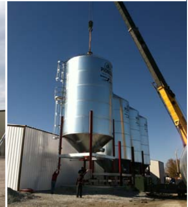
Schuld Bins — Require Crane
