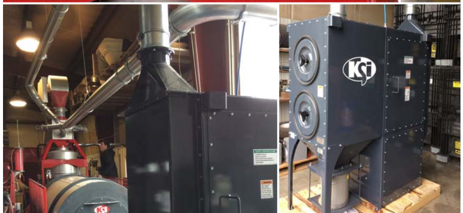
KSi Seed Filtration System Air Handling Unit w/ Collection Bin
